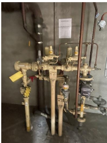
Existing High pressure gas boundary regulator.
