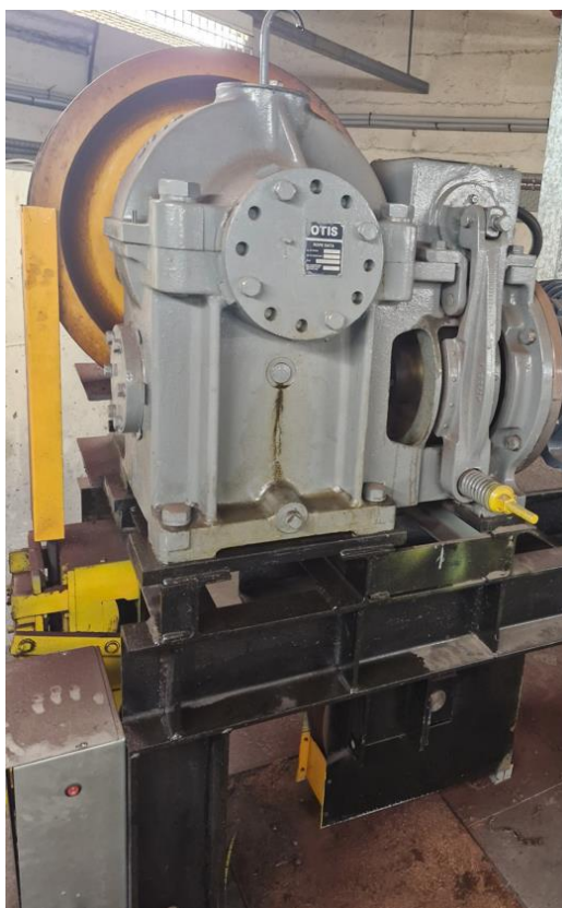
Original as-installed Otis Elevator Geared Machine
