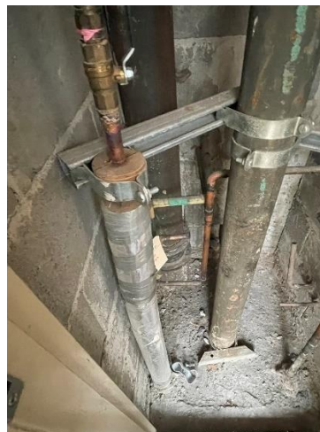
Existing Hot Water services pipework.
