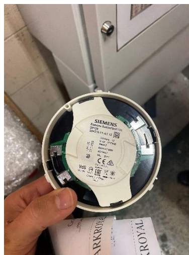
Figure 17: Existing smoke detector.
