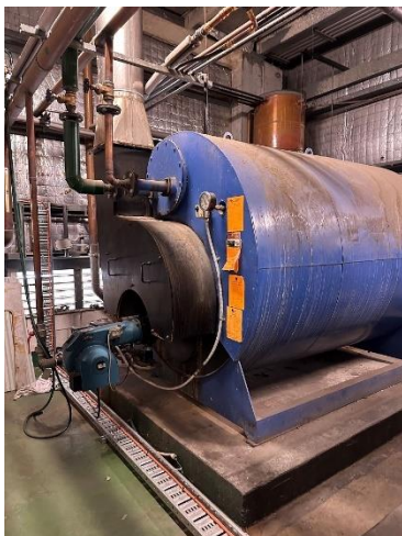
Existing Domestoc HW boiler.
