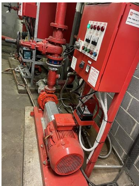
Figure 9: Electric Sprinkler pump
