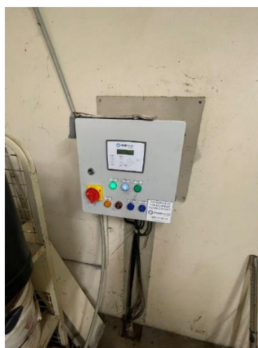
Existing Stormwater pumpstation control panel.
