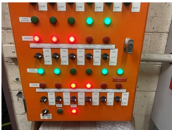
Figure 15: Existing Fire Fan Control panel (FFCP).
