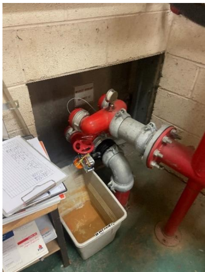
Figure 1: Existing fire hydrant booster assembly
