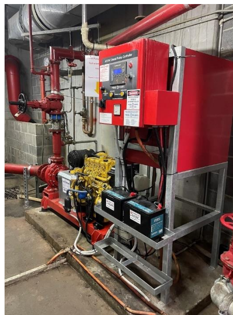
Figure 10: Diesel Sprinkler pump
