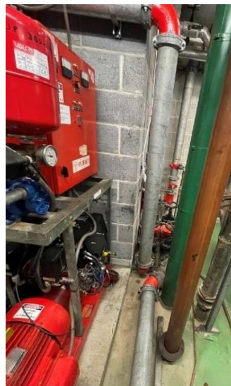
Figure 2: Existing Diesel/Electric Hydrant pump
